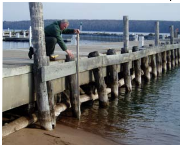
Falling lake levels may make docks and boat ramps unusable.
