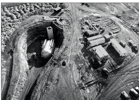
The US Army Corps of Engineers built South Dakota's 15 underground Minuteman missile launch centers in the early 1960s.
